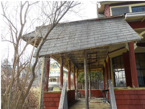
3) Exterior – South/front porch extended overhanging entry porch roof is failing
