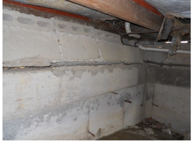
14) Foundation – CMU block courses are tipping, rotating and otherwise failing; large cracks and displaced blocks are present
