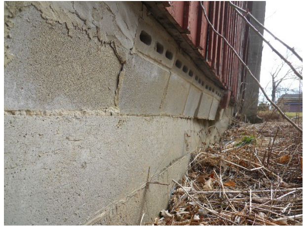
16) Foundation – CMU block courses are tipping, rotating and otherwise failing; large cracks and displaced blocks are present
