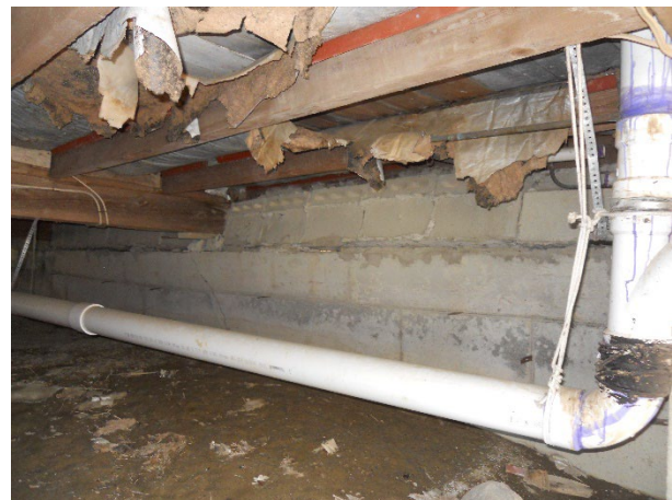
18) Utilities – Main wastewater line runs southerly from north addition to south/front porch where it is disconnected and ends on the ground
