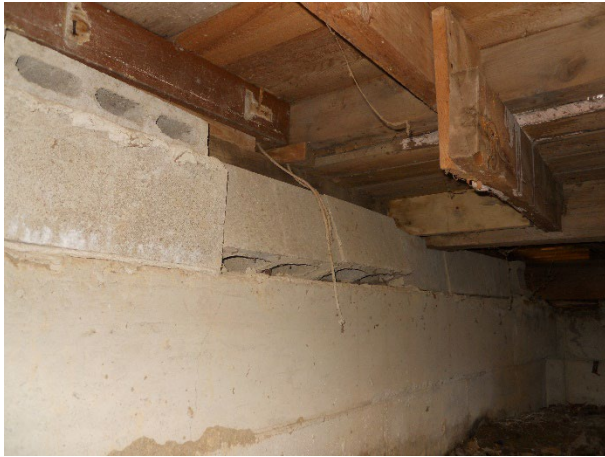
15) Foundation – CMU block courses are tipping, rotating and otherwise failing; large cracks and displaced blocks are present
