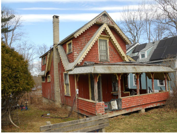
1) Exterior – South/west façades; south/front porch; porch has tarp roof; porch roof and floor are structurally unsound
