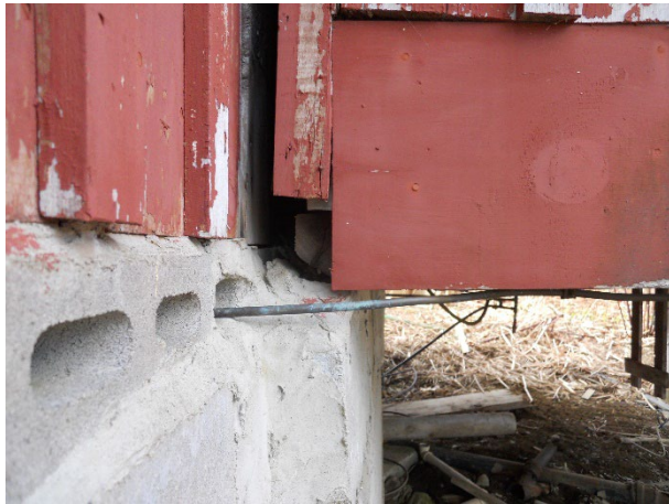
9) Exterior – North addition is separating from the main house
