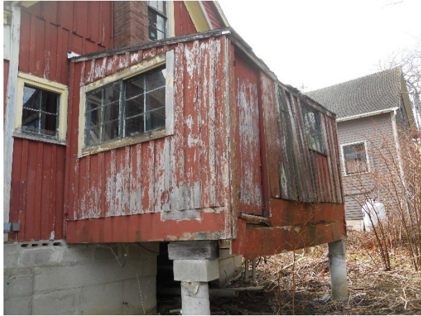
7) Exterior – North addition is degraded and appears structurally unsound
