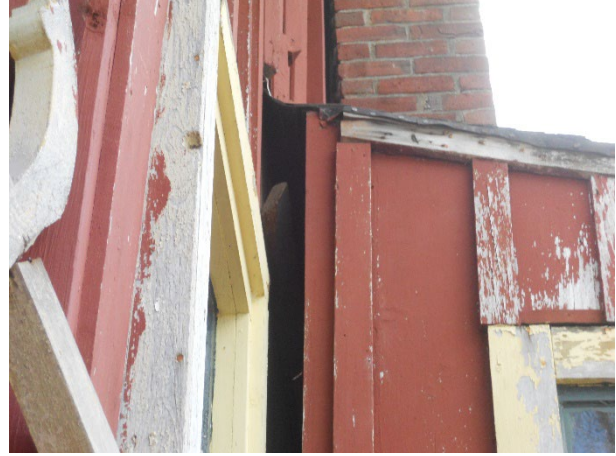
8) Exterior – North addition is separating from the main house; the chimney visible above the addition roof bears on combustible framing
