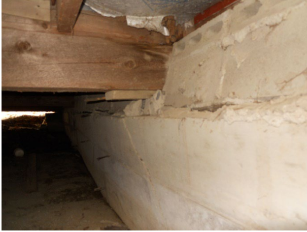
13) Foundation – CMU block courses are tipping, rotating and otherwise failing; large cracks and displaced blocks are present
