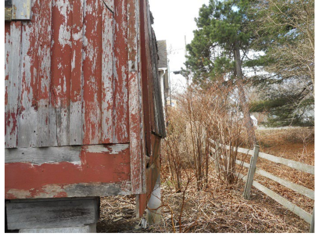
10) Exterior – North addition has significant bulges in the exterior walls, suggesting structural failure in the wood framed walls
