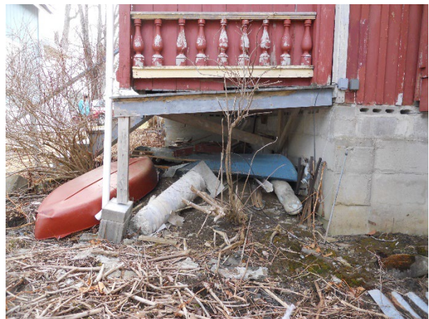
6) Exterior – Northeast corner of northeast porch lacks support; blocks are toppling over (not touching post); floor is deflecting downward
