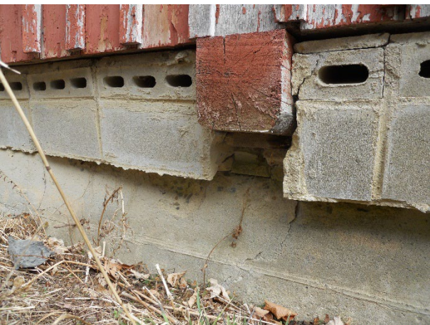
17) Foundation – CMU block courses are tipping, rotating and otherwise failing; large cracks and displaced blocks are present
