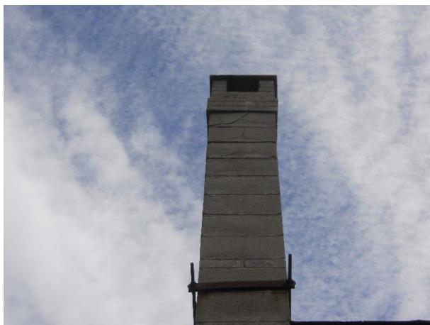
11) Exterior – West CMU chimney has significant cracks and may be unstable above the roof line
