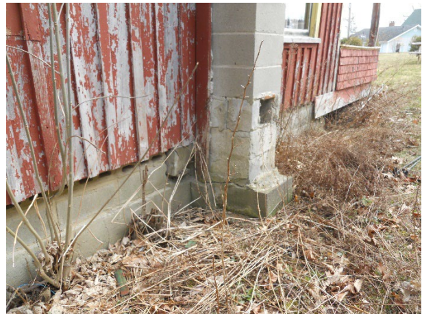
12) Exterior – West CMU chimney has significant cracks and spalling at the base
